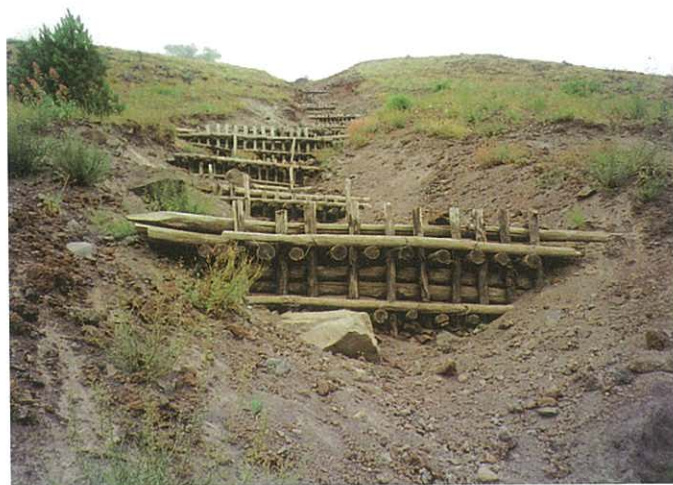
Gully erosion and remedial measures in southern Italy.
